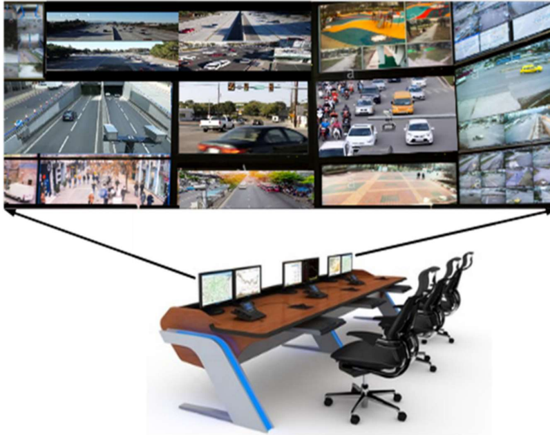
View of manually traffic monitoring at control room.
