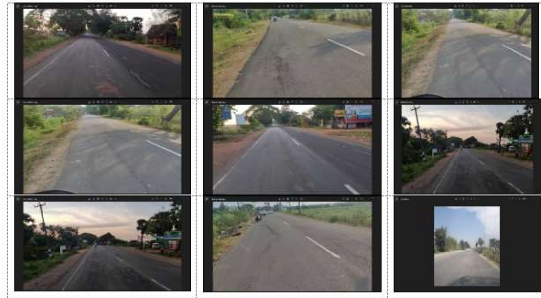
Figure 1. State Highway Road Damage Dataset Sample.
