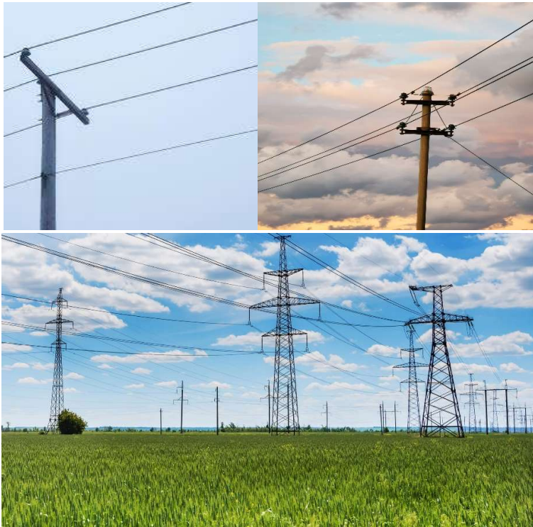
Fig.2 Images of power lines
